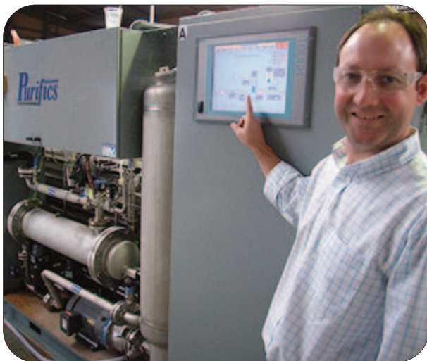
Scott Nairm checks out the groundwater treatment plant at Parafield Gardens.
